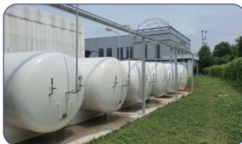
H 2 Supply System
