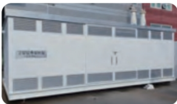
H 2 Compressor Skid
