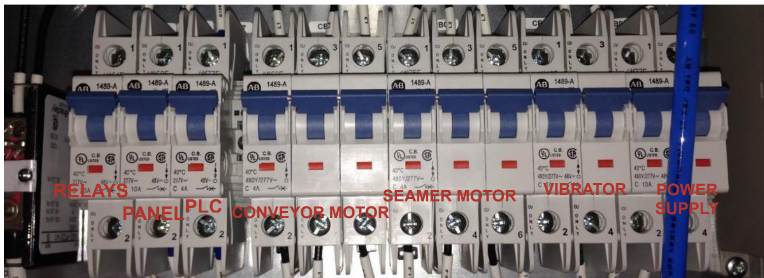
Figure 11 Top row of breakers
