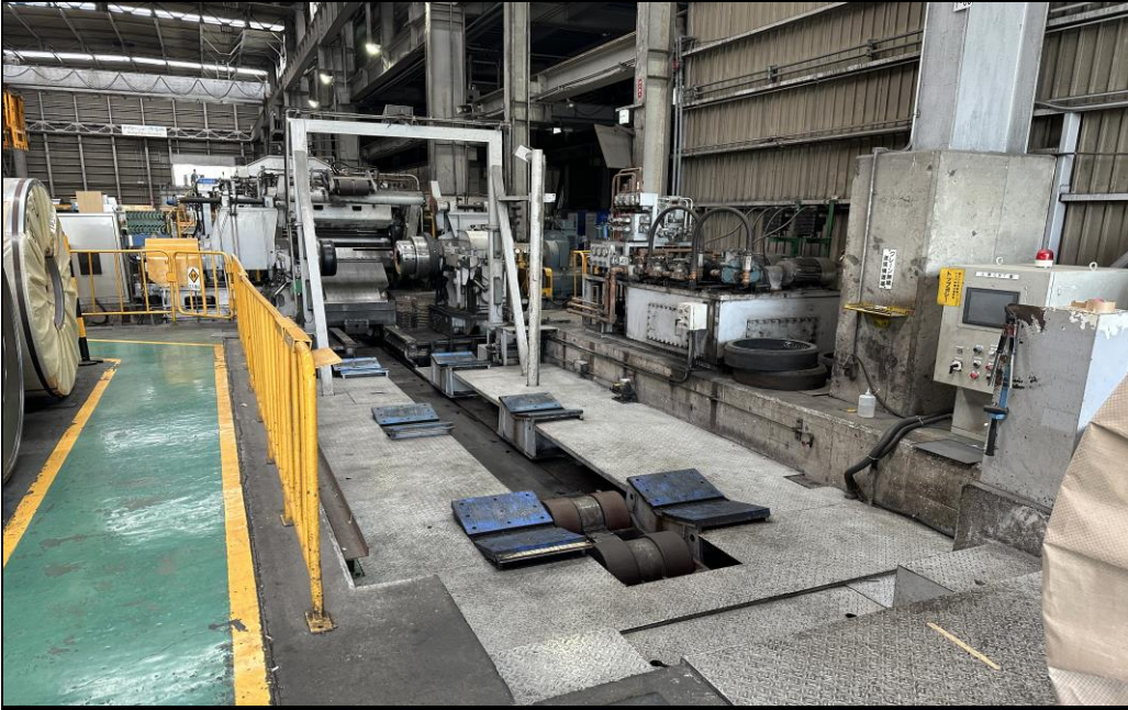
Full View (Entry Side)
