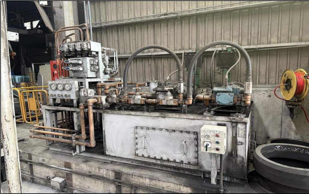
Hydraulic Unit (Entry Side)
