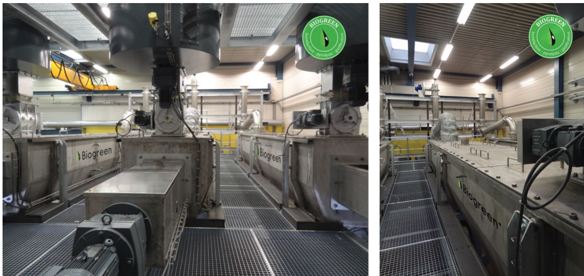
Industrial Biogreen® equipment
