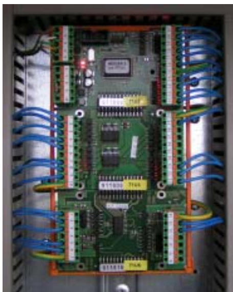
control cabinet line 1b
